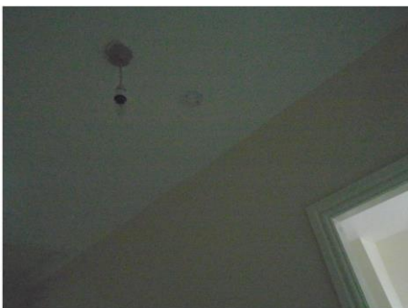
Missing smoke detector
