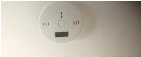
Smoke detector fitted
